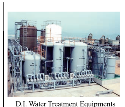
D.I. Water Treatment Equipments
