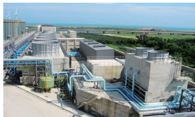
Steel Plant - Cooling Water Circulating Systems
