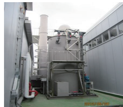
Wet Scrubbers & Ducting
